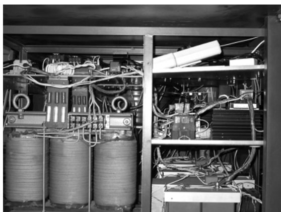
Fig. 2. Power supply external view
